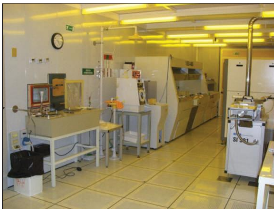
Fig. 20.5 A clean room for lithography usually hosts a self-contained infrastructure. Commonly seen facilities are spin-coater, mask aligner, photolithography stage, lamellar chemical hood, physical vapor deposition unit, microscopes, etc. (reproduced from ref. 7).
